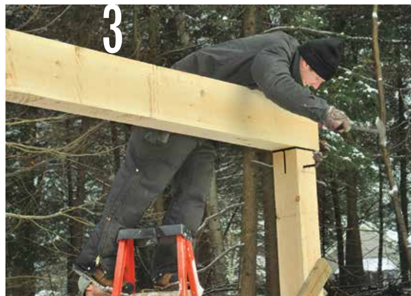
3 Lock the 6×10 plate beam to the 6×6 posts by driving two ½-in.-dia. aluminum pins through the holes at the top of each 6×6 post.
