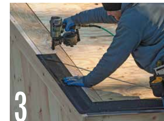
Install starter shingles up each end of the roof, making sure they follow the chalkline. Secure each shingle with 1½-in. roofing nails.
