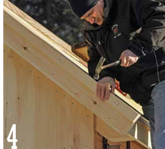
Nail 1×2 trim to the 1×6 rake. This narrow piece of trim isn't required, but it does create an extra shadow line along the gable ends.
