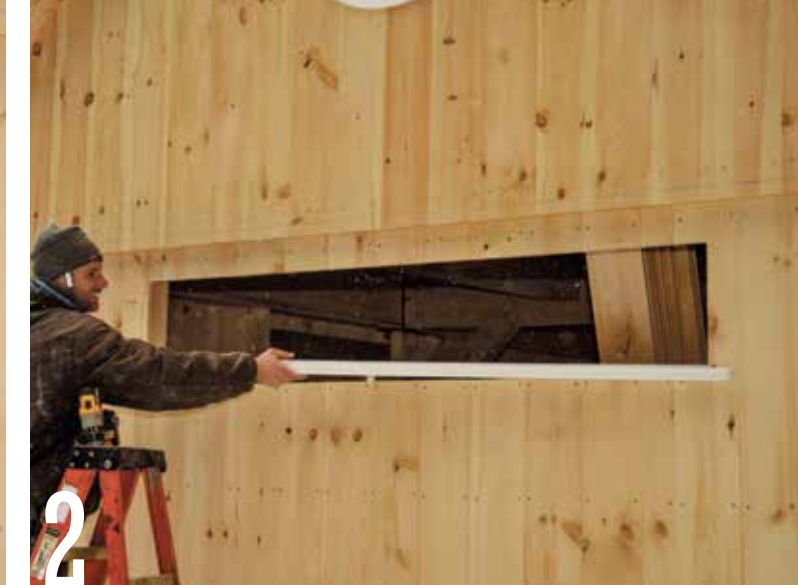
2 Install the PVC windowsill to the bottom of the opening. You could also cut the sill from cedar, redwood, or pressure-treated lumber.
