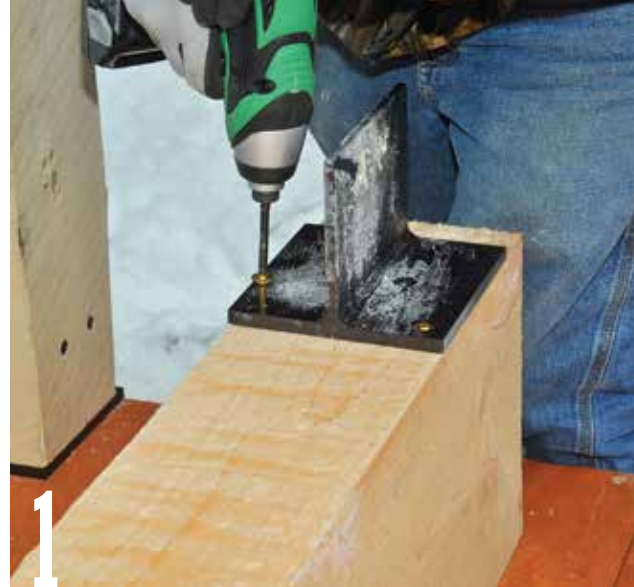
1 Fasten three metal connectors—one for each post—to the edge of the long 6×10 plate beam. Secure each connector with six 4-in. screws.
