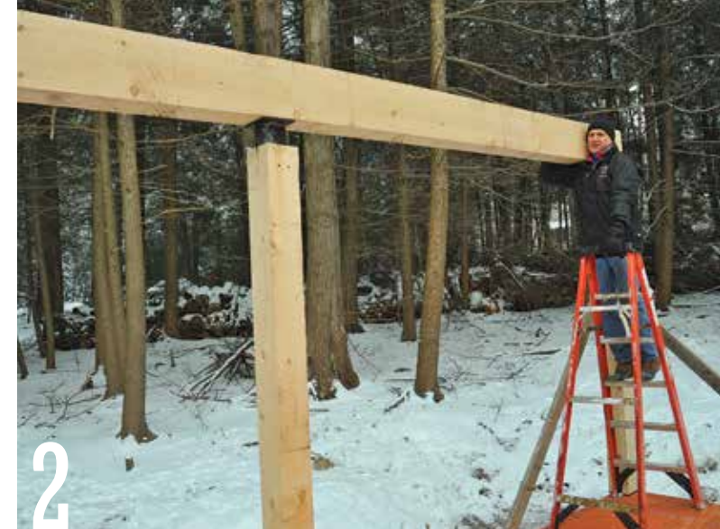
2 Lift the plate beam above the three posts. Lower the beam, guiding the metal connectors into the slots cut in the tops of the posts.
