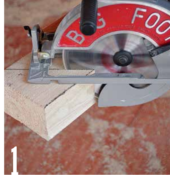
Use a large portable beam saw or 12-in. sliding-compound miter saw to miter-cut the ends of the 4×8 rough-sawn roof rafters.
