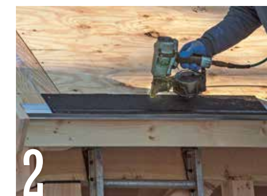
Nail a row of starter shingles along the edge of the roof. Align the top edge of the shingles with the chalkline snapped across the roof.
