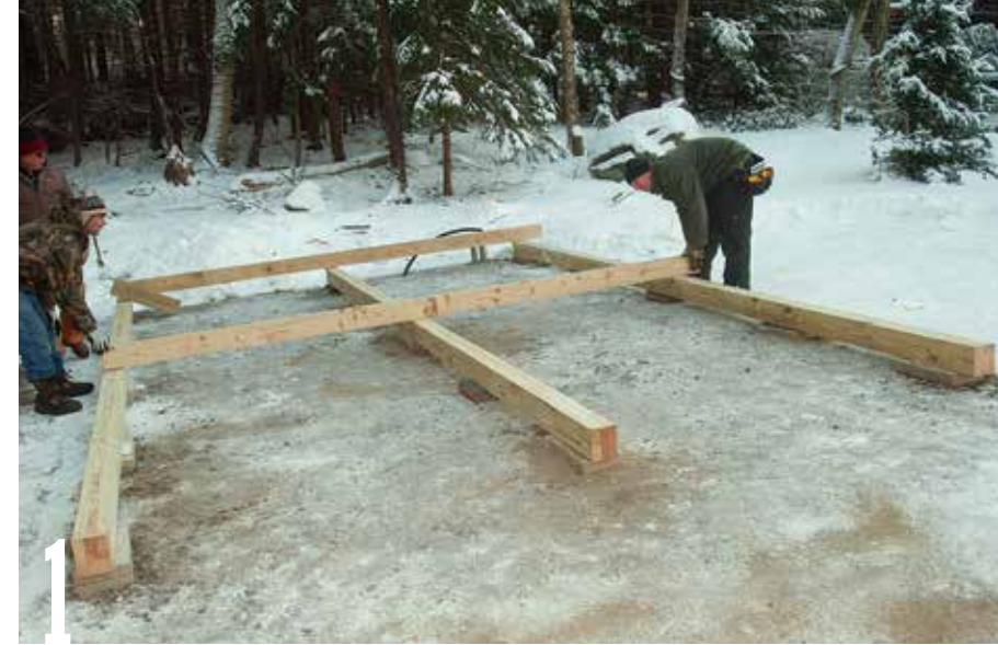
1 Set two 2x6 joists at the far end of the skids, then place another pair in the middle. Cut two more joists for the near end of the skids.
