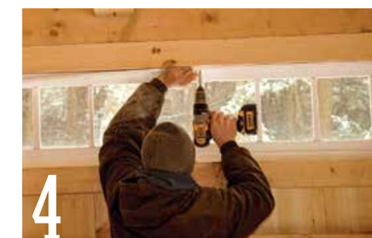
4 Hold the transom window in the opening by attaching a stop strip to the header above the sash. Secure the stop with trim-head screws.
