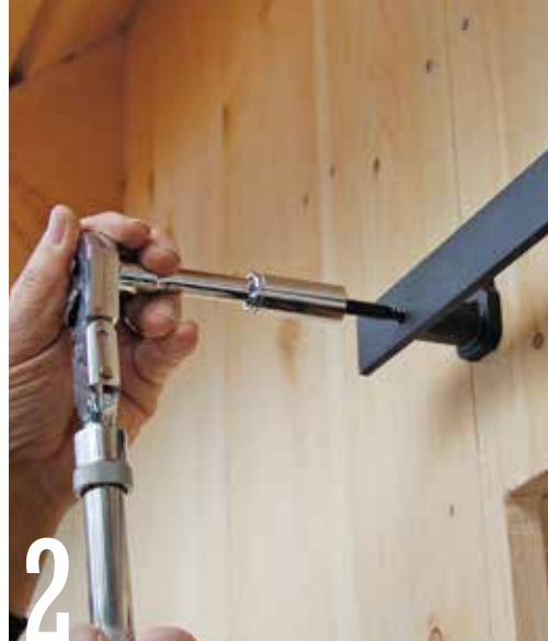
2 Attach the horizontal steel track to each stand-off bracket with a lag screw. Drive in the lags with a ratcheting socket wrench.
