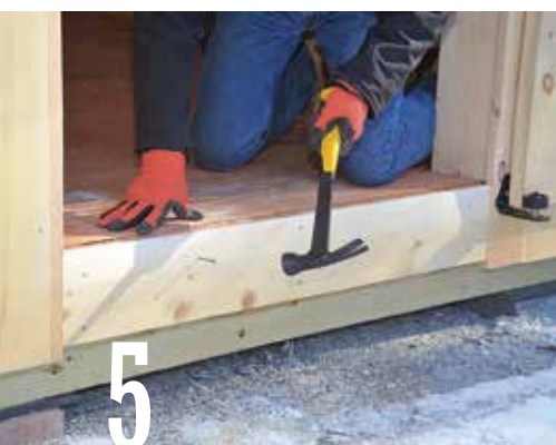
5 Cover the exposed pressure-treated rim joist in front of the sliding door with a pine board. Attach the board with 2 1 / 2 -in. galvanized nails.
