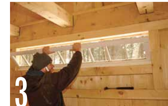
3 Set the transom window on top of the PVC windowsill. Press the window flat against the pine siding that protrudes into the opening.
