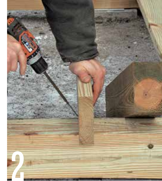
2 Fasten the 2x6 joist to each of the three skids with a 3-in.-long decking screw down at an angle and into the top of the skid below.
