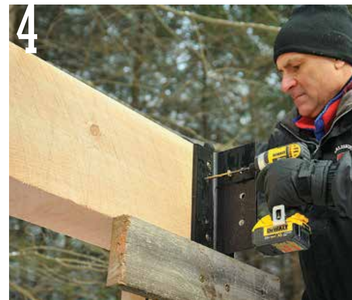
4 Screw a 24-in.-long temporary 2×6 cleat to the posts and then set a metal T-Rex connector on top of the cleat. Fasten the connector to the 6×10 plate beam with six 4-in.-long structural screws.
