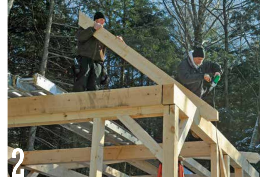
Hold a roof rafter in place and secure its lower end to the top of the 6×10 plate beam with two 10-in.-long structural screws.
