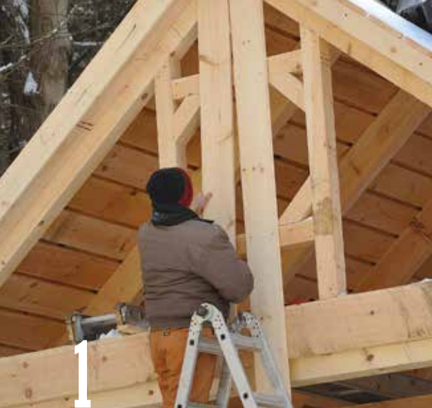
1 Start installing siding in the middle of the gable end. Spline together the two center boards, so the tongue edges are facing out.
