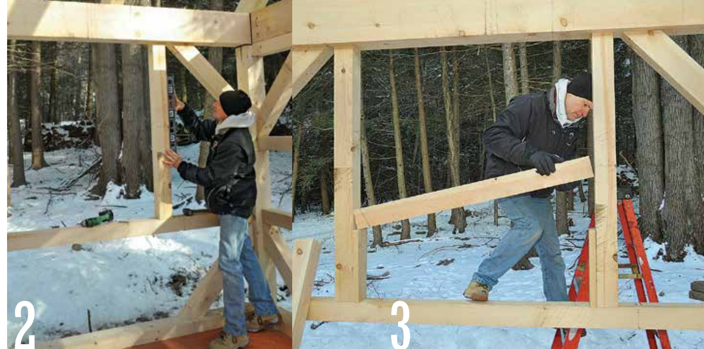
2 Frame the sides of the window openings with 4×6 trimmer studs. Check each 4×6 for plumb with a level before screwing it in place.
