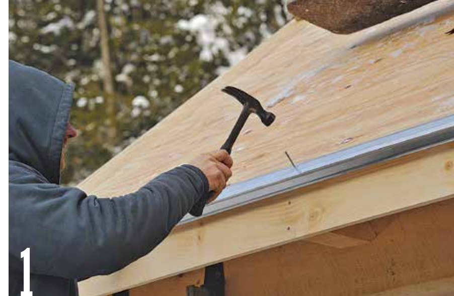
Set the aluminum drip-cap flashing onto the roof edge, positioned so that its wide flange lays flat on the plywood deck. Secure to the roof with 1½-in.-long nails.
