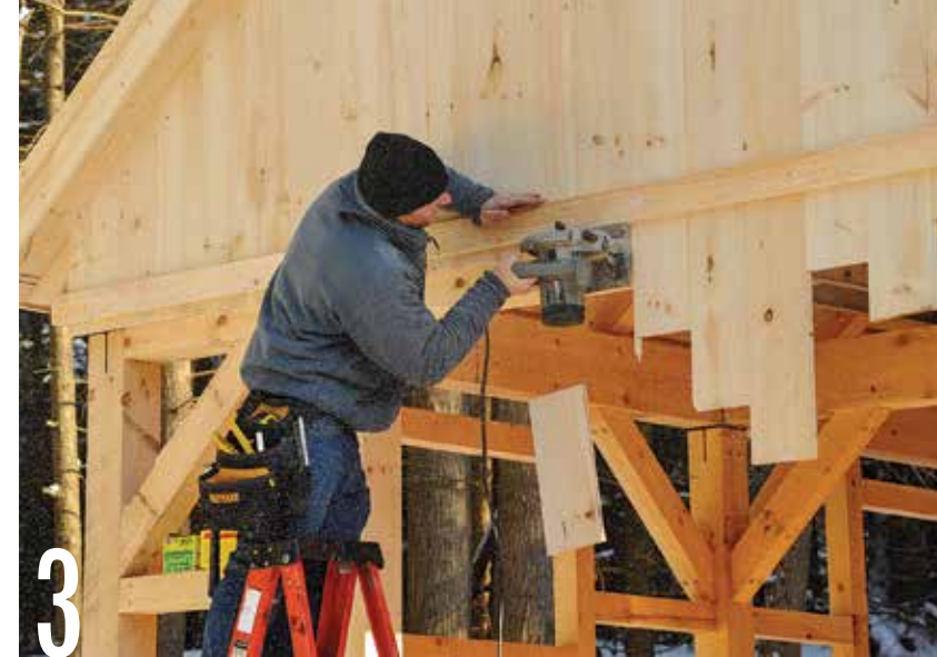
3 Adjust the sawblade to cut 1/8 in. deep, then guide a circular saw along the 2x4 fence to trim the siding to length. Unscrew the 2x4.
