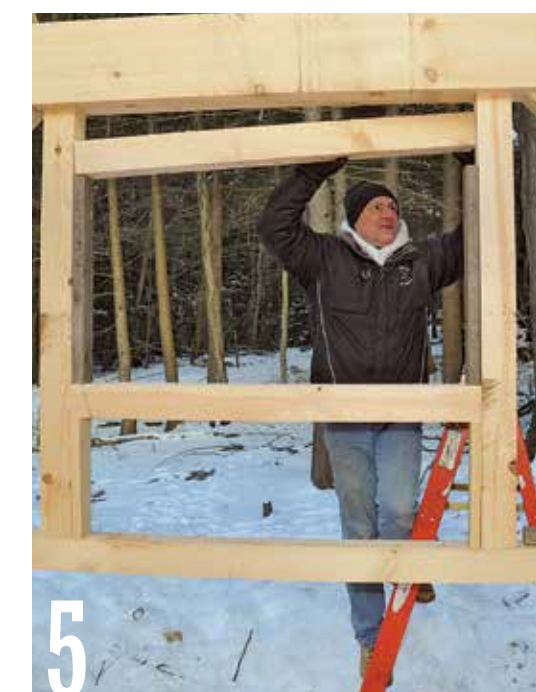
5 Saw a 4×6 header to fit between the vertical trimmer studs. Push the header down onto two 25-in.-long spacer blocks, then secure with 6-in. screws.
