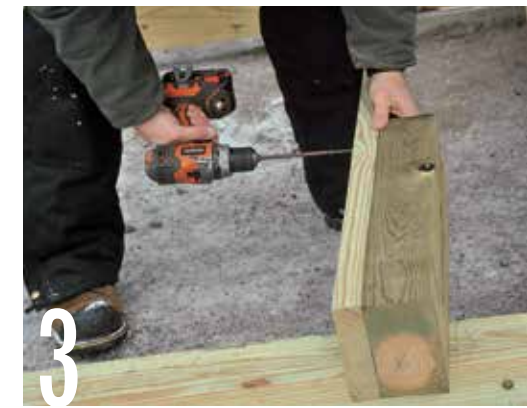
3 Hold a 24-in.-long support block of pressure-treated 4x6 against the inside of the joist. Drive 3-in. screws through the joist and into the block.
