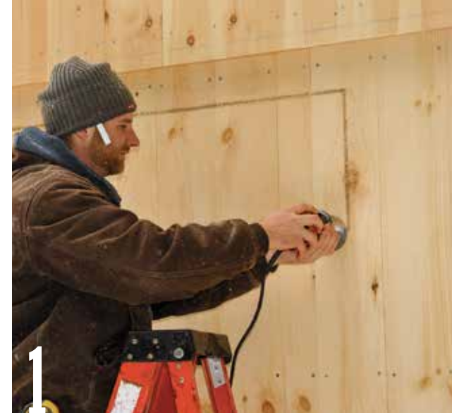
1 Turn on the router and then slowly move it in a clockwise direction to cut through the siding around the window's rough opening.
