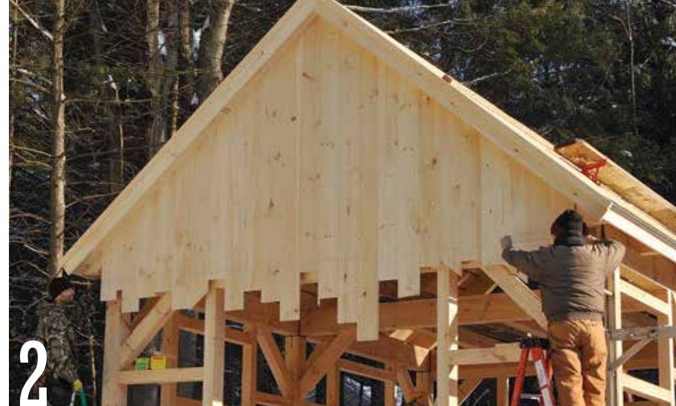
2 Snap a chalkline across the jagged ends of the siding. Then screw a long, straight 2x4 fence to the siding, flush on the chalkline.
