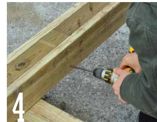
4 Place another 2x6 floor joist against the opposite side of the 4x6 block and secure it with 3-in.-long galvanized decking screws.
