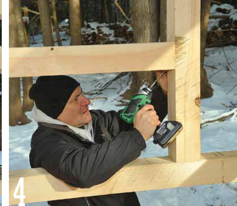
4 Drive a 6-in. screw through the outside of the sill and into the trimmer. Move the spacer block and drive two screws up from below.
