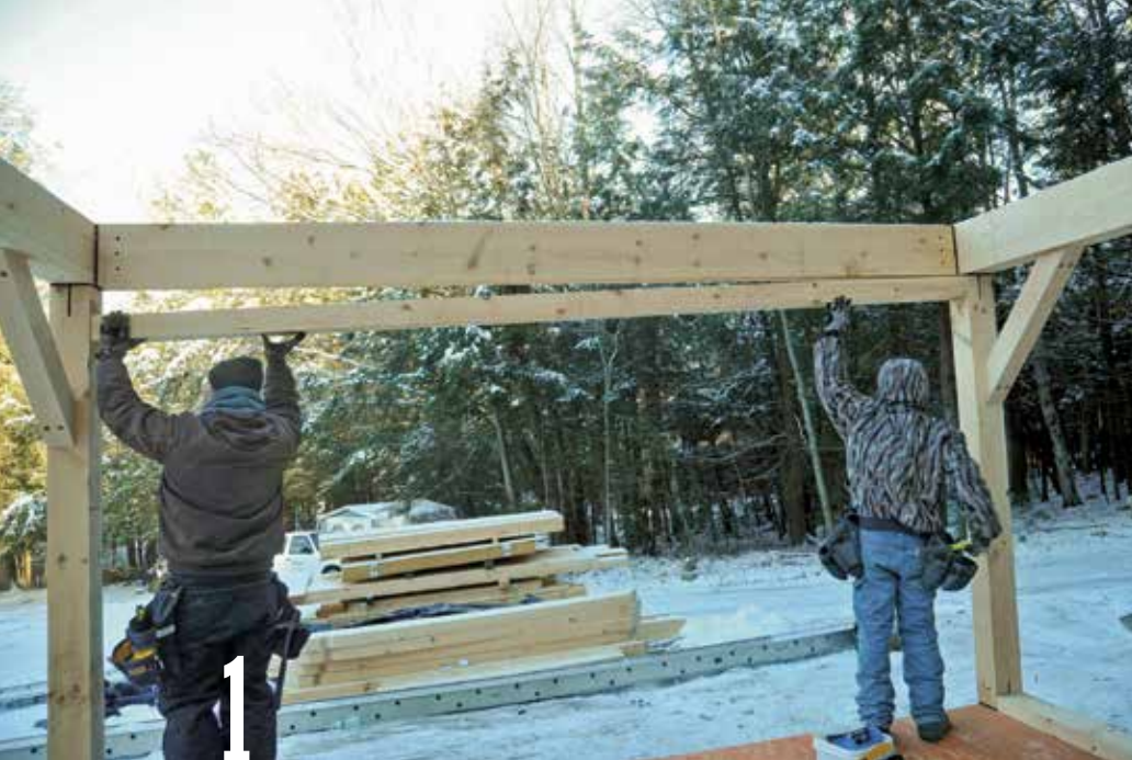
1 Use 8-in. screws to fasten a 4×6 nailer to the underside of each 6×10 crossbeam. Hold the nailer flush with the outer surface of the beam.
