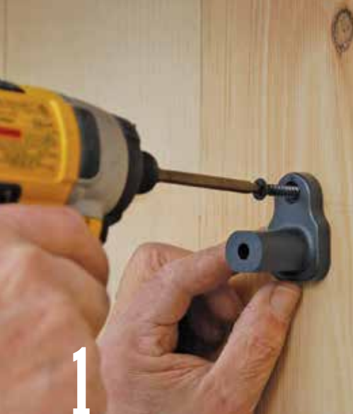
1 Fasten five iron stand-off brackets to the barn directly over the doorway opening. Mount each bracket with a single screw.
