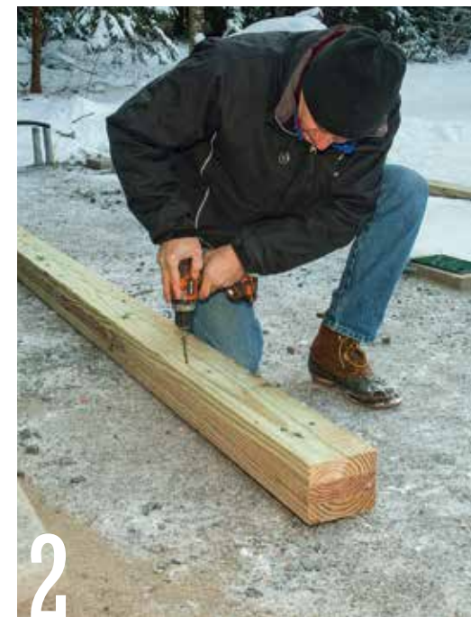
2 Make each 20-ft.-long skid by screwing together three pressure-treated 2×6s. Drive the 3-in. screws in from both sides of the skid.
