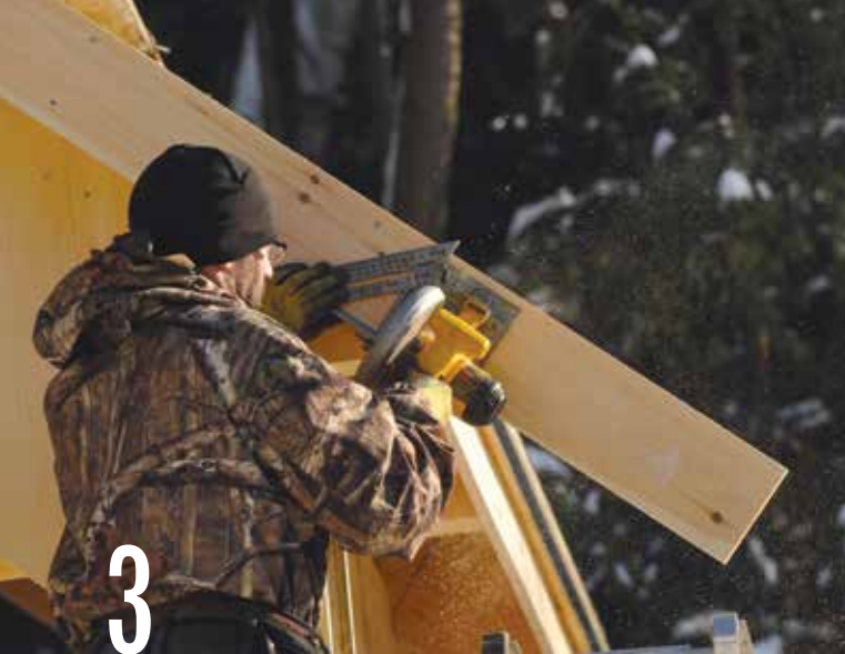
Cut the 1×6 rake board longer than needed, then nail it to the fly rafter. Use a circular saw to trim the rake flush with the fascia board.
