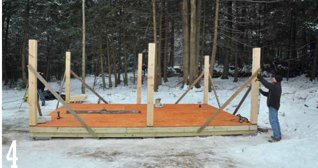
4 Temporarily hold the posts plumb with diagonal 2×4 braces. Fasten the braces to the floor frame and posts with 3-in. screws.
