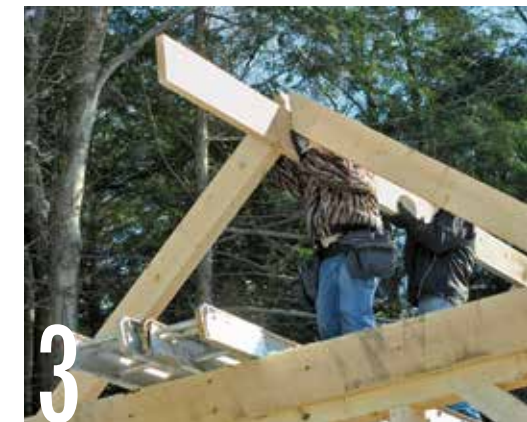
After installing two pairs of rafters, slide the 2×10 ridge beam between the rafters. Be sure the ridge is flush with the tops of the rafters and secure each rafter to the ridge with two 6-in. screws.
