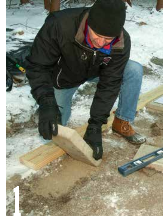
1 Set the solid-concrete blocks into place, then check them for level. Use a long, straight 2×6 to align each row of five concrete blocks.
